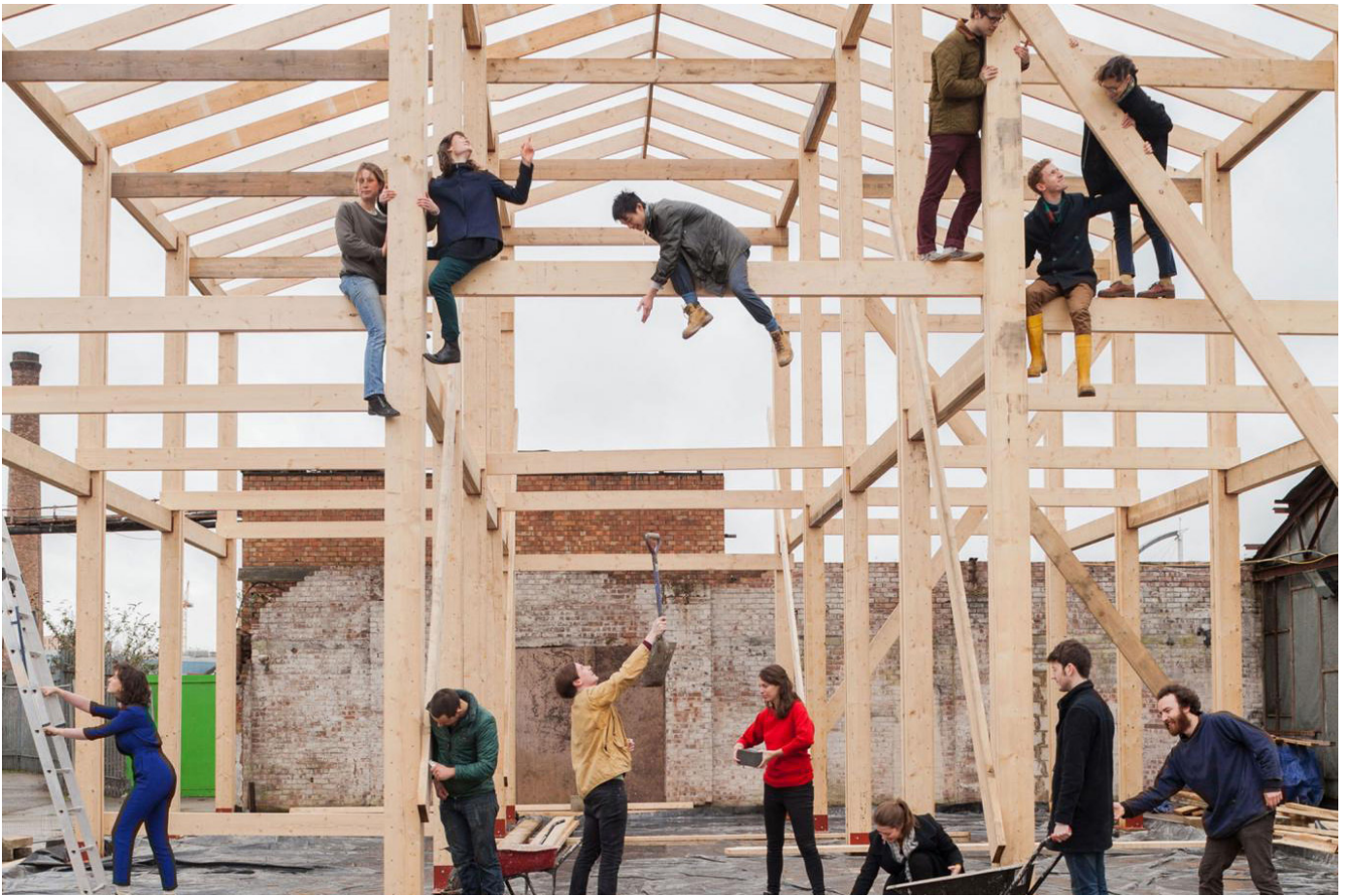
Above : Yardhouse project images (top: concrete tile detail, bottom: frame under construction)
